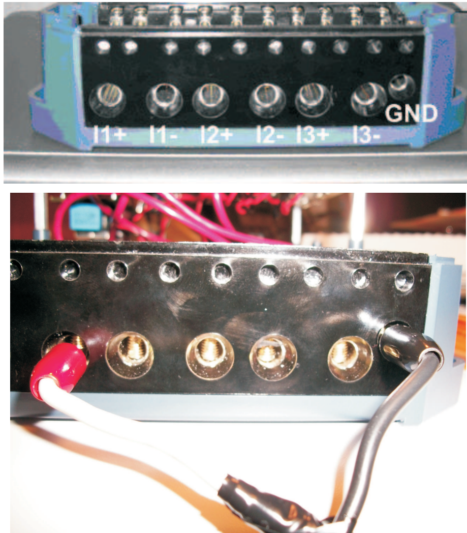
Figure 8. Power Strip Connector to Energy Meter
