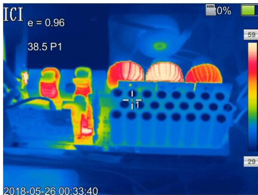
Figure 76. Thermal Image of the TIDA-01604 at 240-V AC Input With 6.6-kW Load
