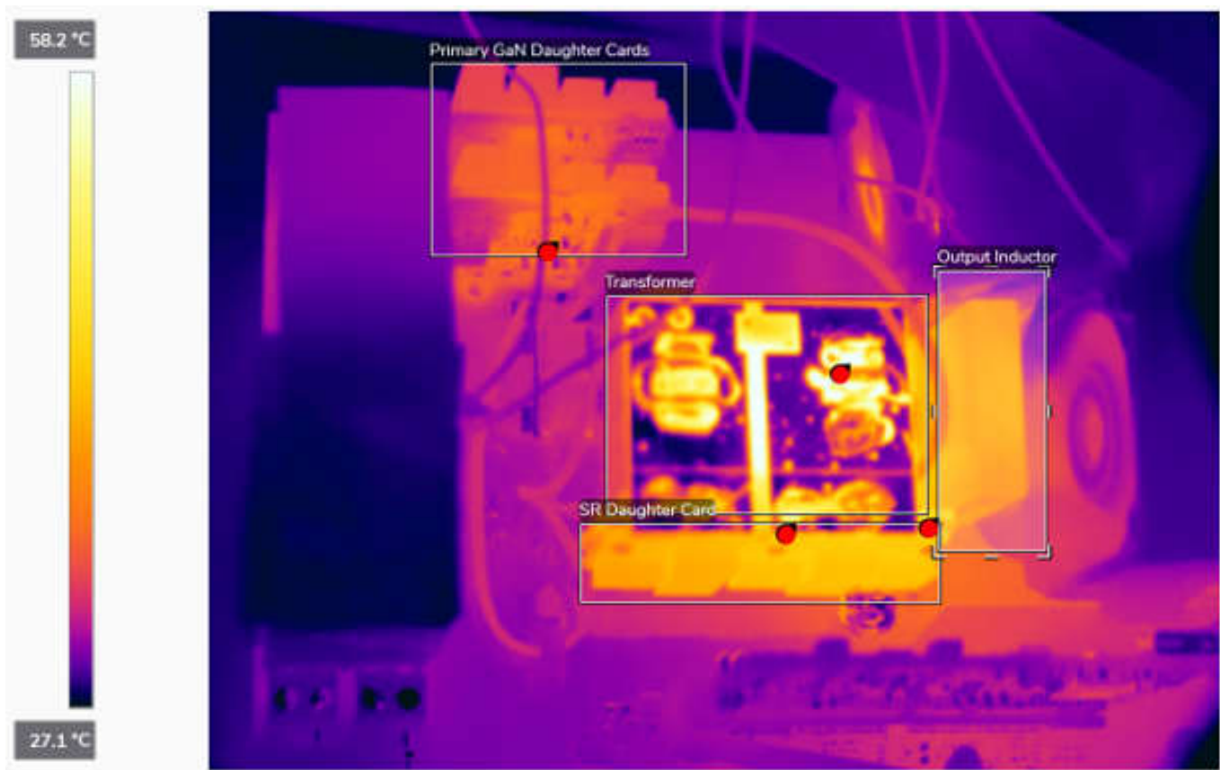
Figure 2-2. 3-kW Thermal Image
