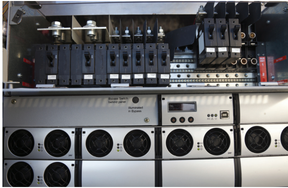
Figure 1. A modular telecommunications power system.
